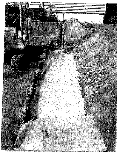
5. Gravel provides extra capacity, filter fabric protects gravel from mixing with backfill. Both are optional per manufacturer.
